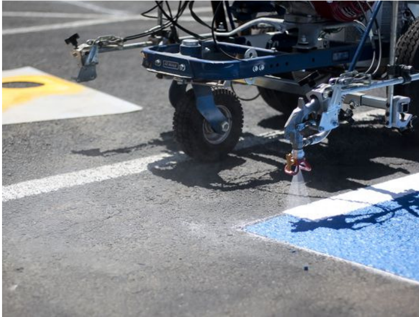
Nick Tetzloff, 19, of Chandler, restripes the lot at Y Knot Party Rentals in Mesa on July 14, 2016. The business is restriping the handicap stalls in their parking lot to meet accessibility requirements outlined by the Americans with Disabilities Act. (Photo: Charlie Kaijo/The Republic)
